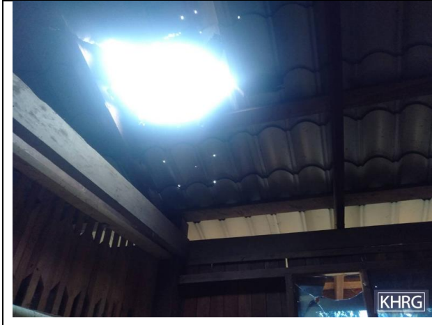
This photo was taken on January 9 th 2022 in H--- village, Yo Klah village tract, Bilin Township, Doo Tha Htoo District. This photo shows the roof and window of a villager’s home that were damaged by SAC mortar fire. [Photo: KHRG]
