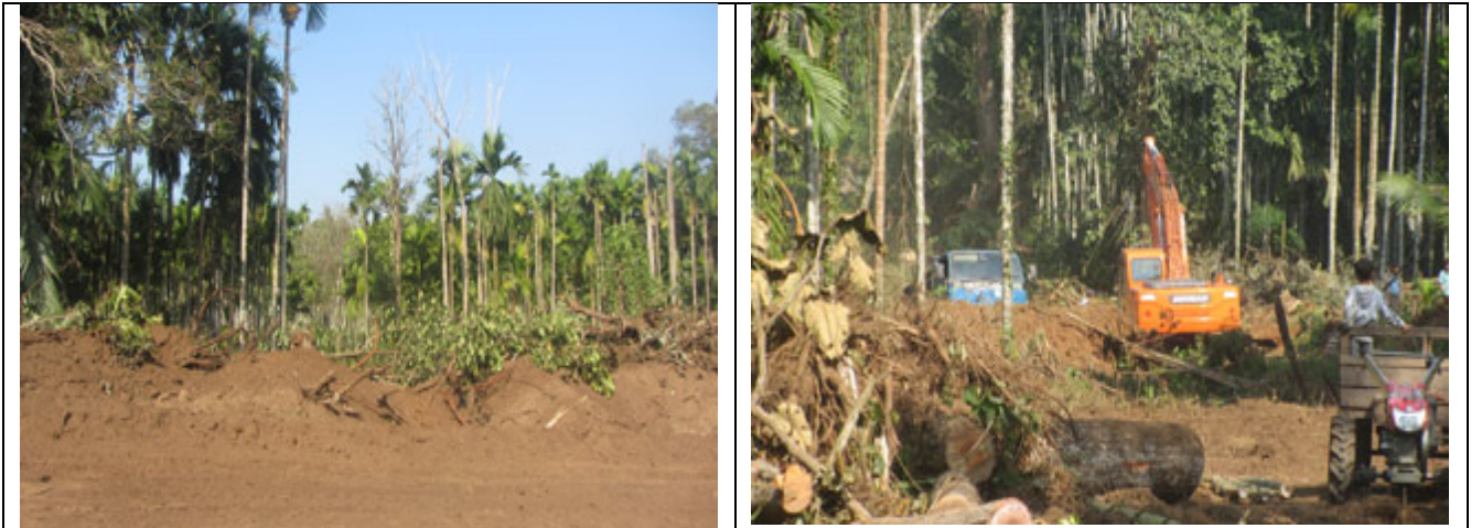
These photos showing road construction occurring between Law Pa and A'Kluh village were taken on December 10 th 2013 in Kawkareik Township, Dooplaya District. The photo on the left depicts the harm done to a coconut grove due to the construction. The photo on the right shows heavy machinery clearing the community's coconut plantation to construct the road. The road will connect Kawkareik and Kyonedoe townships and has negatively impacted villagers' livelihoods due to the loss of land and destruction of agricultural products. [Photos: KHRG]
